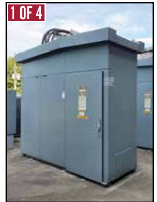
SQUARE D Primary & Secondary Disconnects
