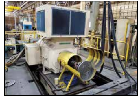
1,000-HP Dynamometer Motor Test Stand
