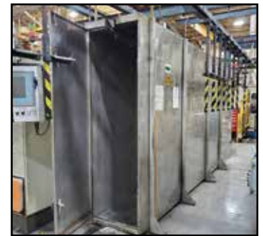
Armature Overhead Trolley System
