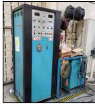
HI-POTRONICS Transformer Unit
